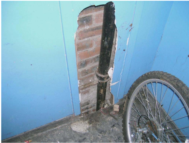
Figure 6.4 Asbestos insulating board; consideration should be given to removal as the board in this location is vulnerable to damage
