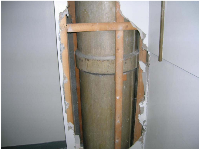
Figure 4.2 Asbestos insulating board boxing partially removed to show asbestos cement flue pipe behind.
