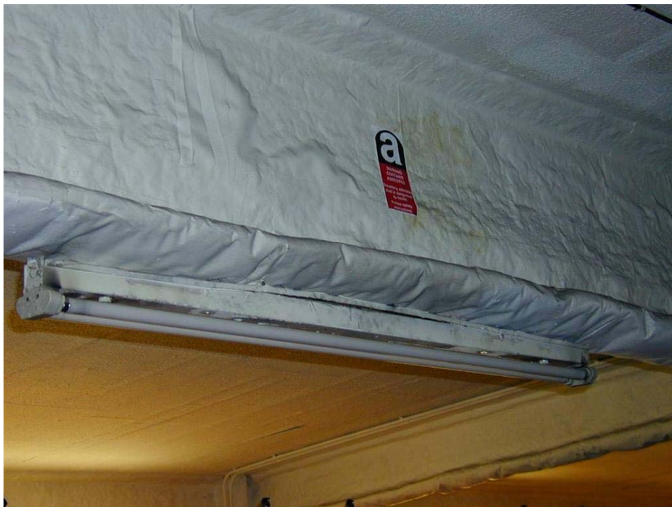
Figure 4.11 Asbestos insulation on structural steel.
