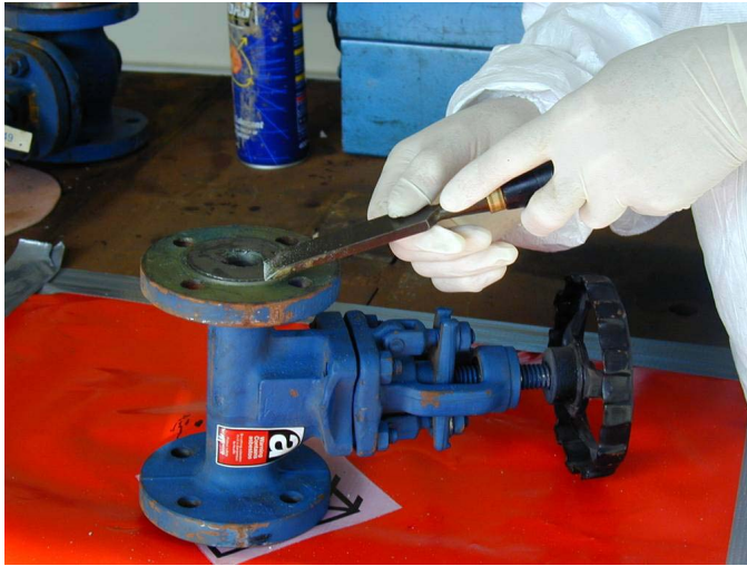
Figure 11.5 Use of hand tools only to clean asbestos gaskets and residue from a valve.
