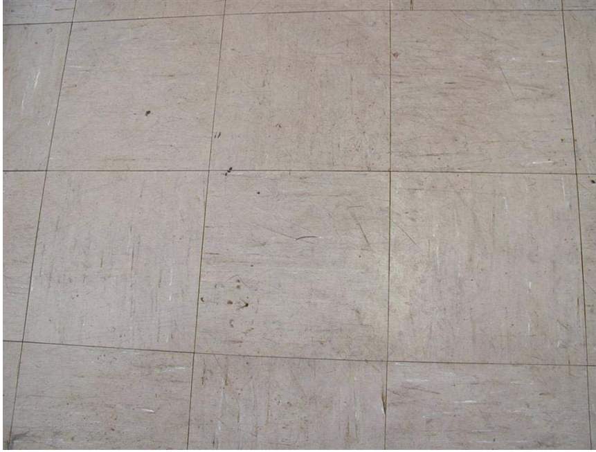
Figure 4.6 Asbestos floor tiles
