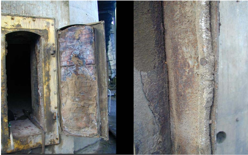
Figure 4.12 Asbestos rope sealing on chimney door. The image on the right is a close up view of the rope.
