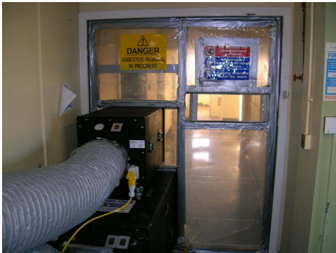
Figure 12.2 Negative pressure units and air discharge ducts, viewing panels and warning signs.
