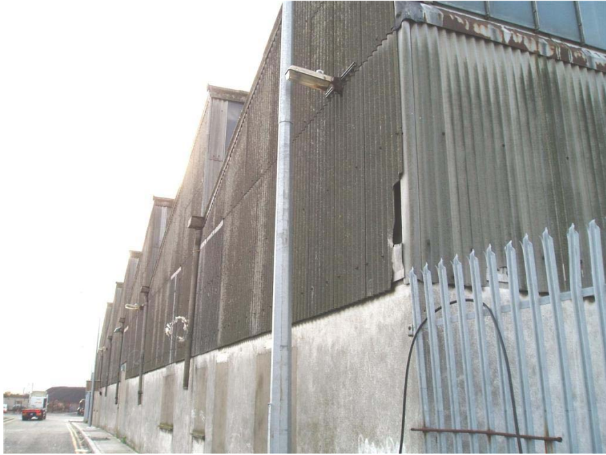
Figure 4.10 Asbestos cement cladding on a factory
